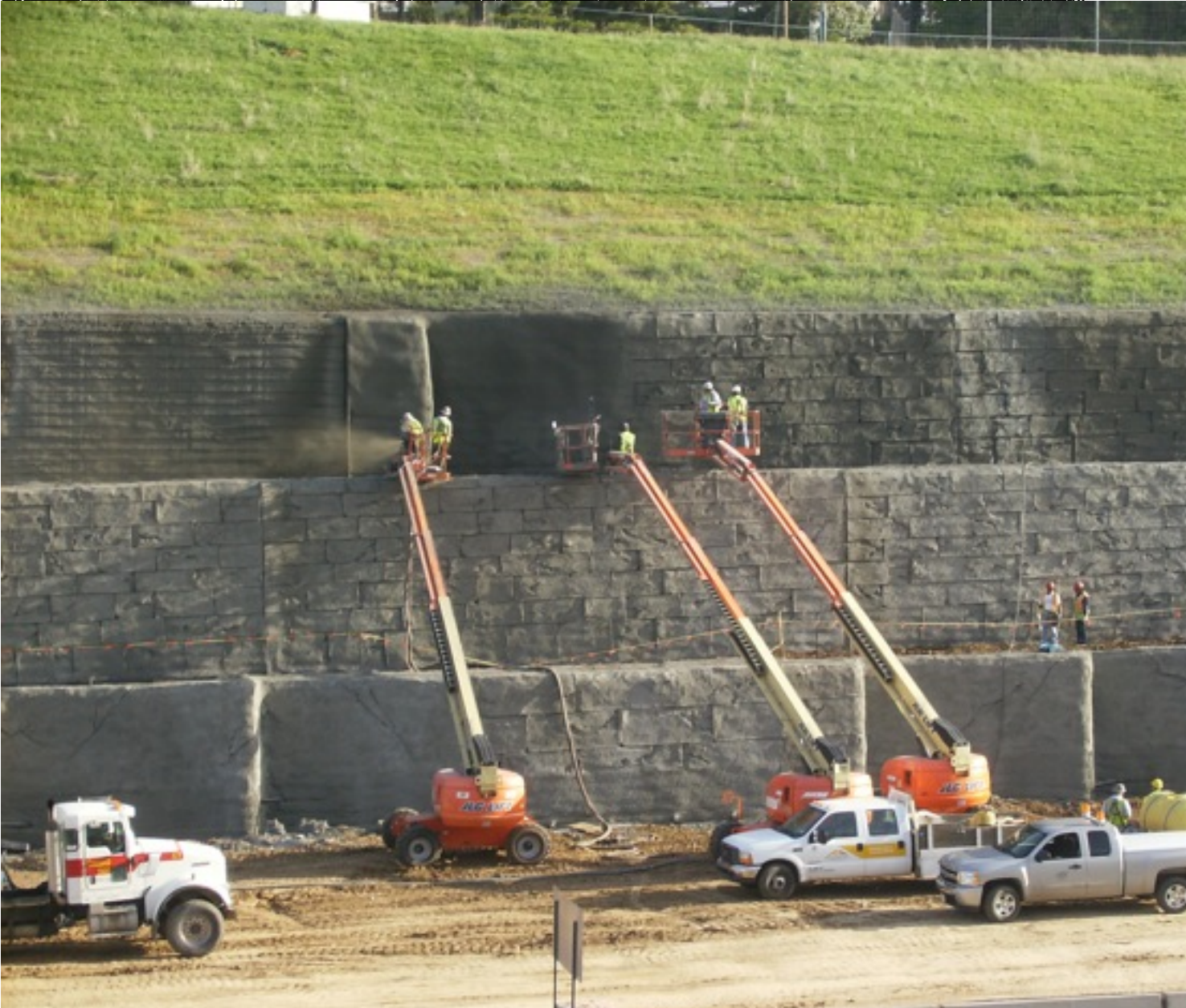
The soil nail wall was installed and constructed by the contractor. The project was completed by the contractor.
